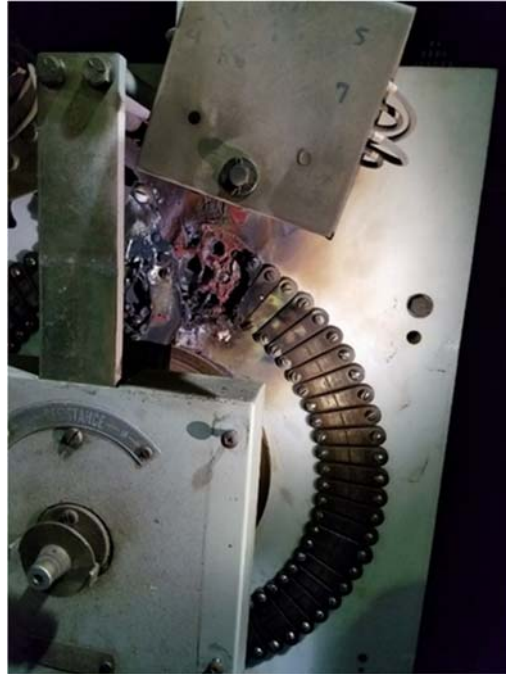
Figure 16 Damage to Field Rheostat
